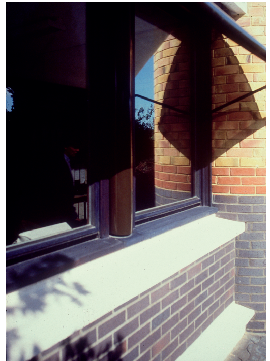
The simple 'butcher's blinds' were controlled with sophistication. They kept out the sun while allowing a clear view out. More than dumb Hi-Tech louvres do!
